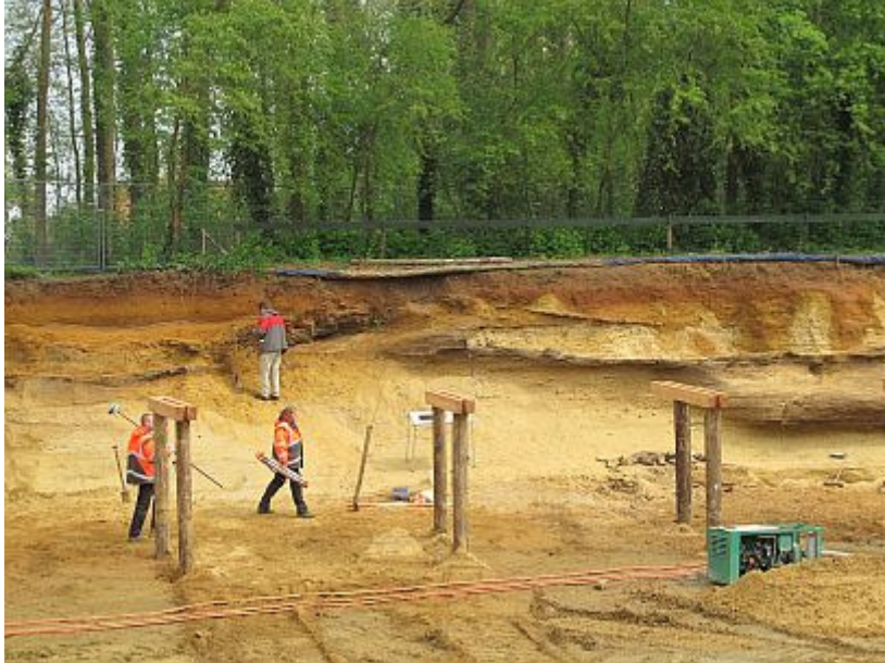
Research during construction work. This geoheritage site is made accessible to the public.
